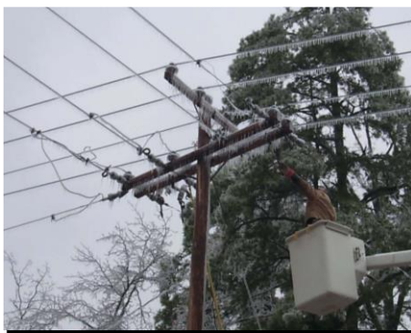
December 2000, Statewide ice storm. Utility workers repair damage to Pine Bluff Arsenal distribution system
